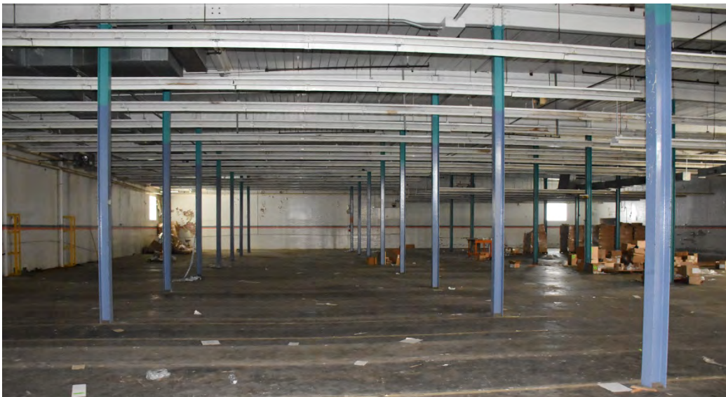
Late 1950s addition second floor looking northwest (top), 1937 addition first floor looking south (center) and second floor looking west (bottom)
